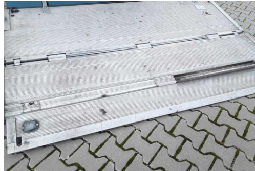
Abrollsicung LBW defekt
